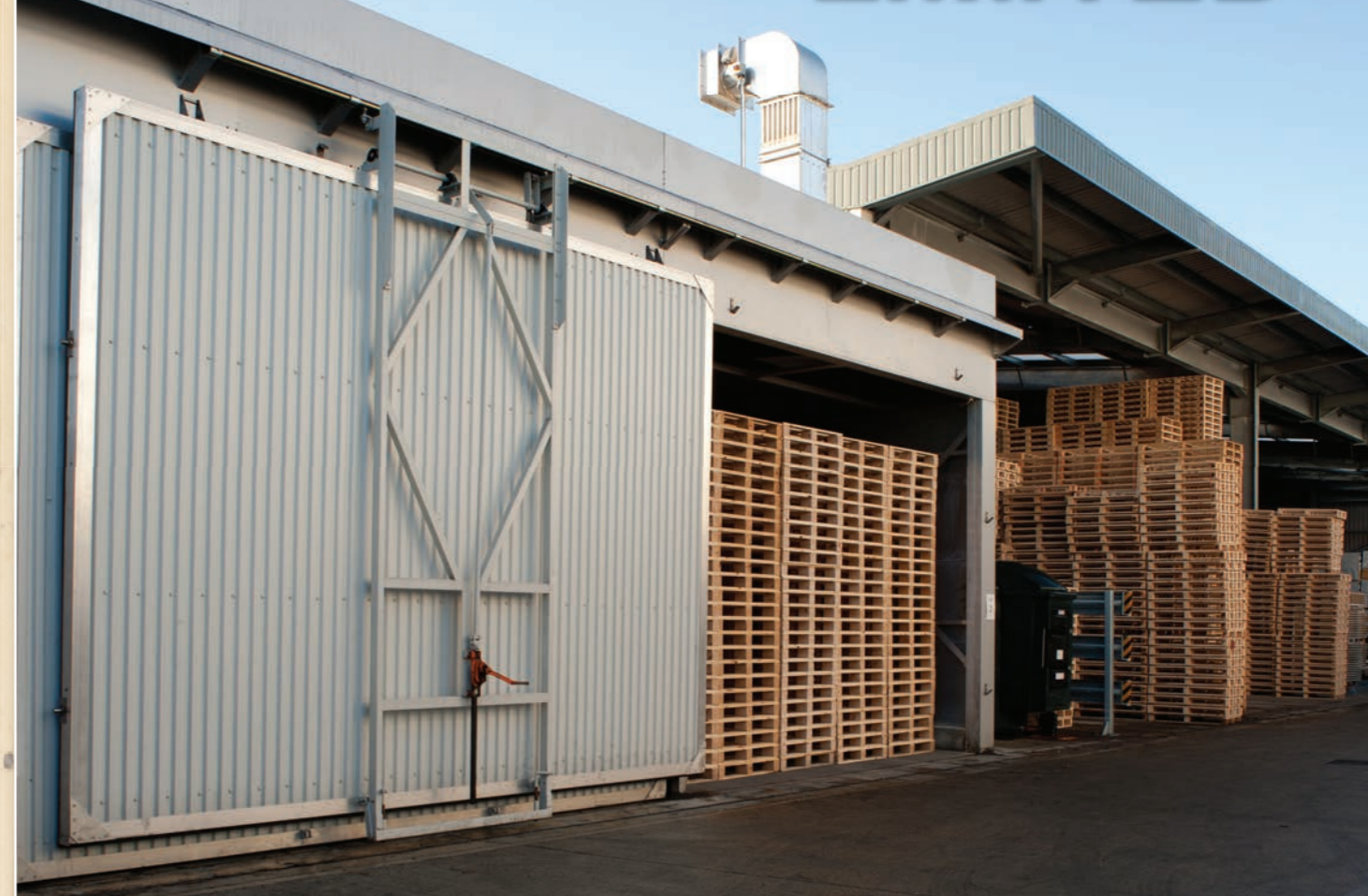
2 kilns with the capacity of 700 Euro pallets each
